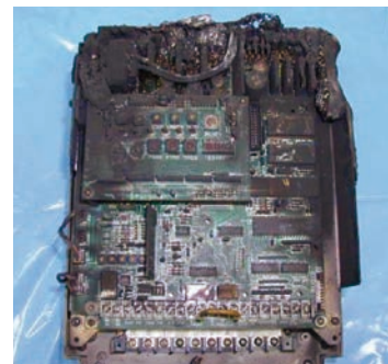
Burnout of the AVR control section caused by contamination
