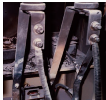
PT burnout caused by insulation deterioration
