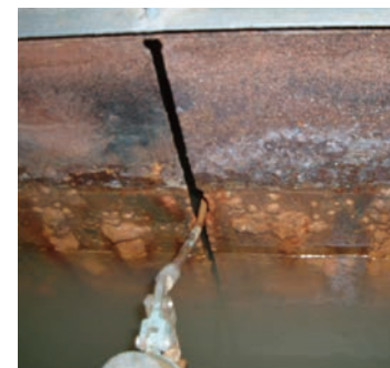
Corrosion in the cooling water tank
