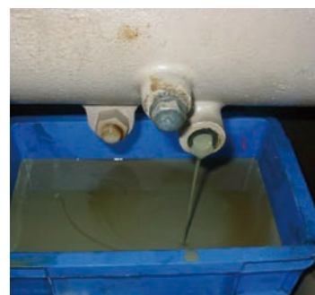
Emulsification of the lubricating oil caused by the entry of cooling water
