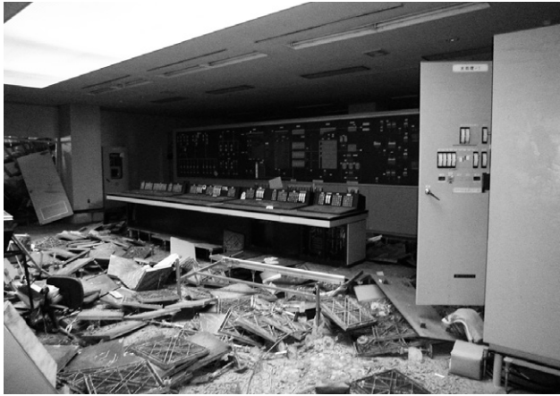
Fig. 4 Situation of Damage in the Control and Monitor Room at the Kesenuma WWTP
