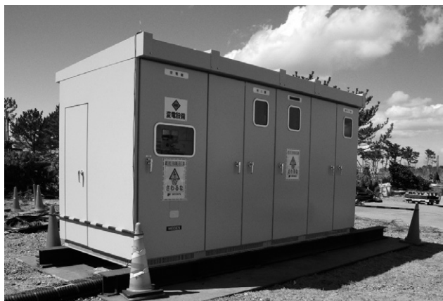
Fig. 1 Temporary Outdoor Incoming Substation Facilities at the Kennan WPC
