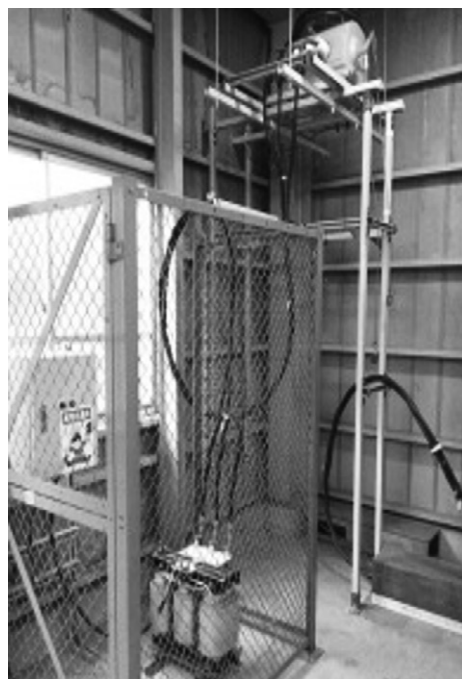
(b) 6kV voltage step-up facility
