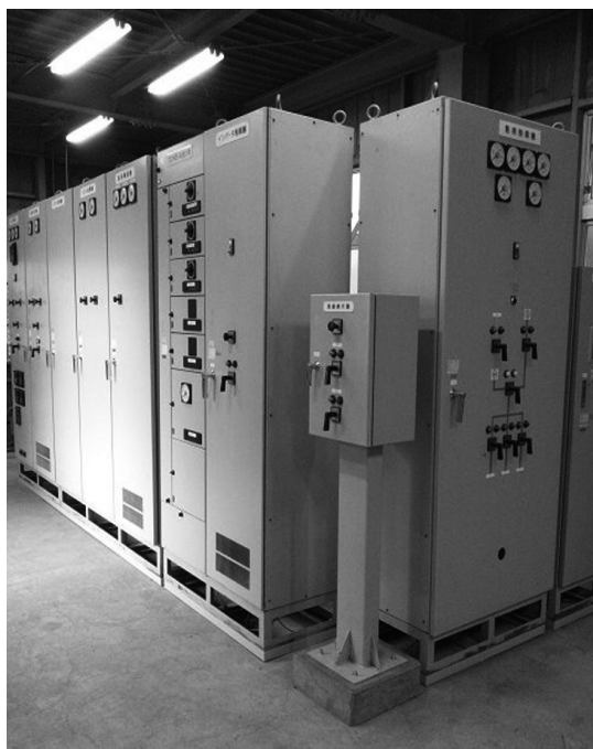
(a) Distribution panel
