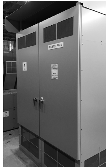
Fig. 4 Resistor Panel for Maintenance
