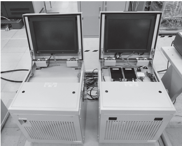
Fig. 3 On-Board Equipment inside Train
