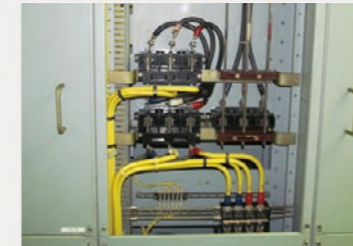
Measuring position: MCCB
