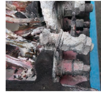
Burning out of a tap changer on a motor transformer by the looseness with vibration
