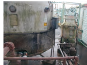
Adoption of inverters for air-conditioner pumps
