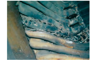
Stator winding ground fault in a cage-rotor type induction motor
