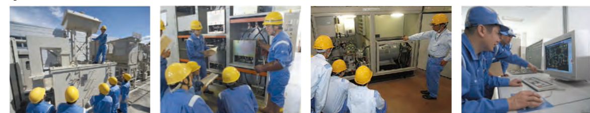
High-voltage (66kV) power receiving substation system
