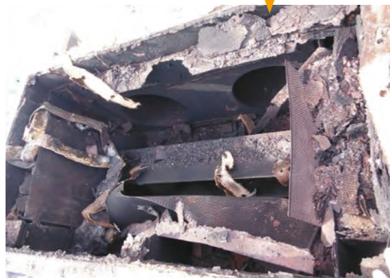
Lower part of an exhaust duct
