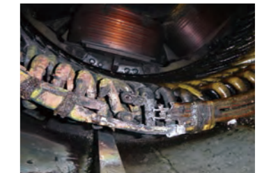
Burnout of a stator winding of a regular-use engine generator
