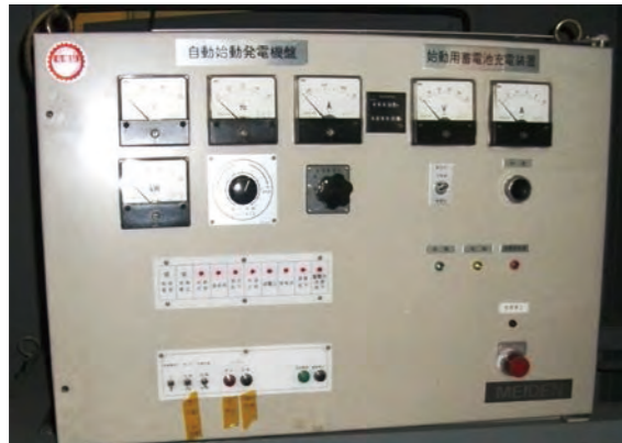
Old panel before renovating
