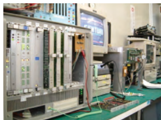
Control rack (Power source and IC boards) repair and life extension services
