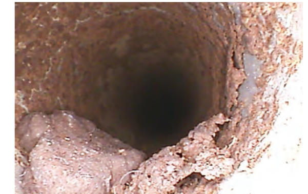
Inside of generator air cooler piping
