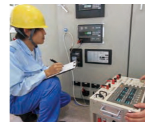
Characteristic test of protective relay
