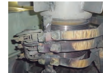
Burnout of a current collector of a wound-rotor type induction motor
