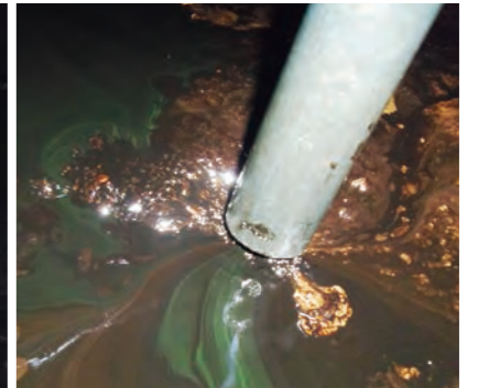
Sludge accumulated in the underground tank
