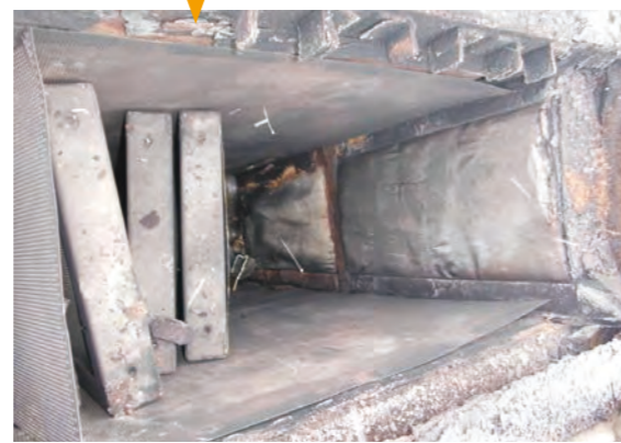
Mid-section of an exhaust duct
