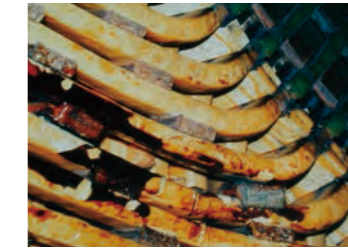
Stator winding ground fault in a steam turbine generator
