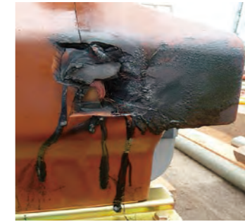
Burn-out due to ageing degradation of VT
