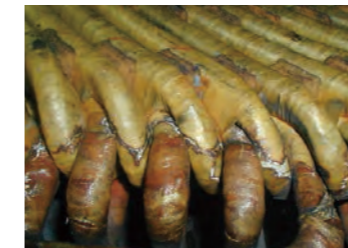
Tracking in stator winding of a cage-rotor type induction motor
