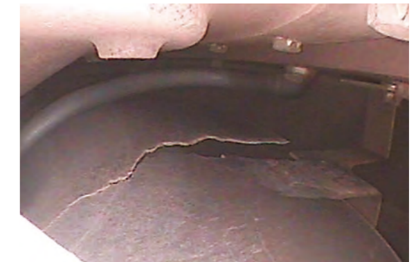
A crack inside a gas turbine
