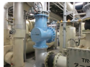
Improvement of refrigerator efficiency
