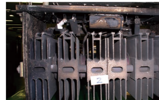
Burning of a thyristor unit (fouling)
