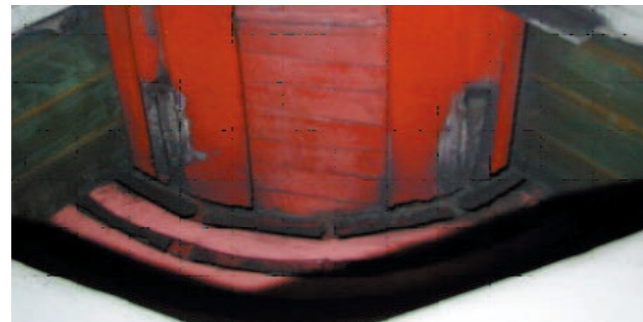
Transformer with insulation breakdown
