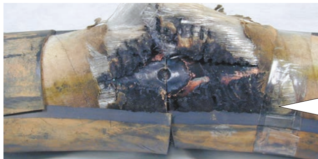
High-voltage cable with insulation breakdown
