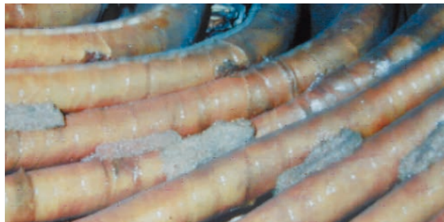
Insulation breakdown of electric motor stator coils
