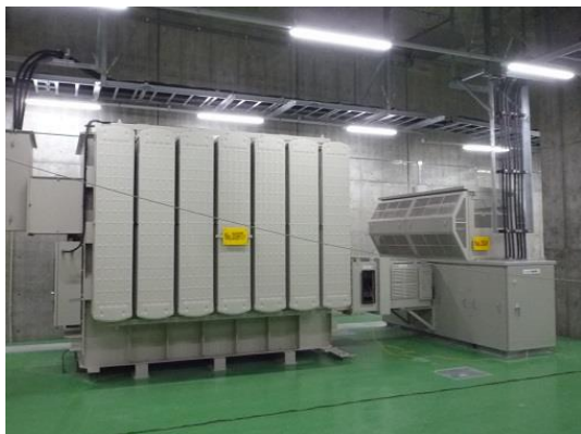
Transformer for a rectifier (left) and a silicon rectifier (right)
