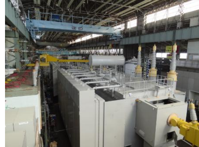
Current state of the transformer factory testing facility
