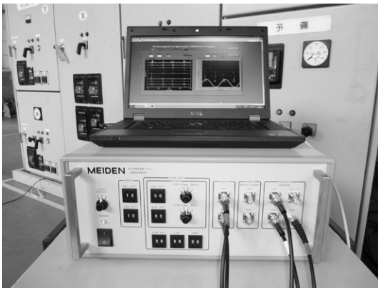
(b) Partial discharge measuring equipment by the electromagnetic detection method
