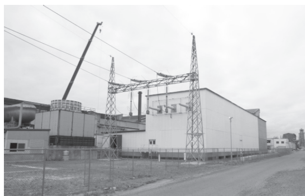
Fig. 7 Restored Power Receiving Substation
