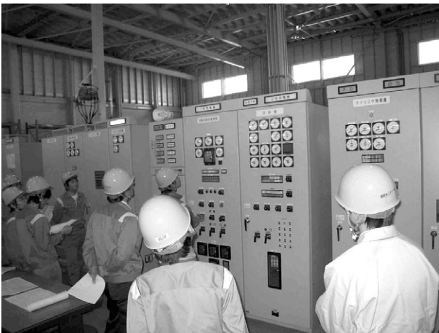
Fig. 13 Training for Power Generation Facilities (Auto-Start Generator Panel)
