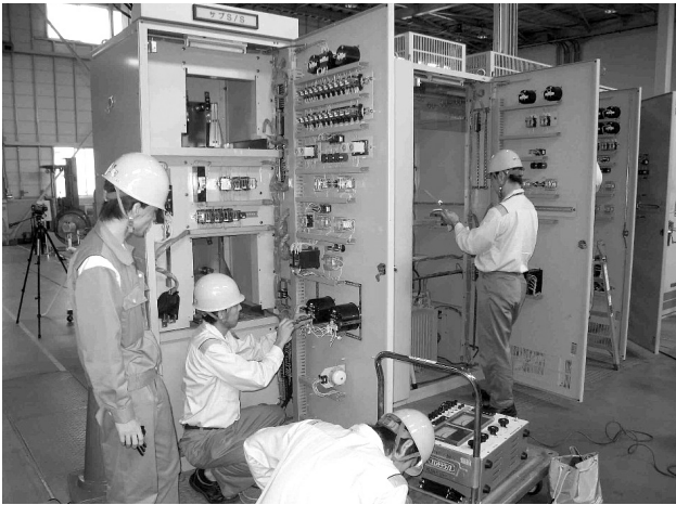
Fig. 4 Inspection Training for High-Voltage Substation Facility
