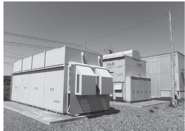
(a) Sodium sulfur battery
