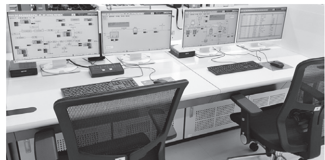
Fig. 1 View of Installed Monitoring Terminal
