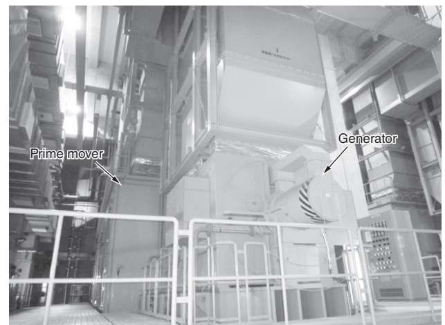
Fig. 1 23 MVA In-house Emergency Power Generation System
