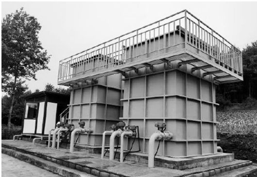
Fig. 8 Distributed Water Purification Facility in China
