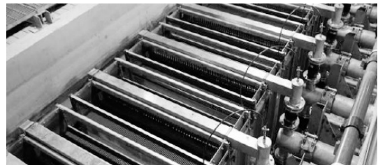
Fig. 12 Ceramic Flat Sheet Membrane Unit of Water Purification Facilities in Saudi Arabia
