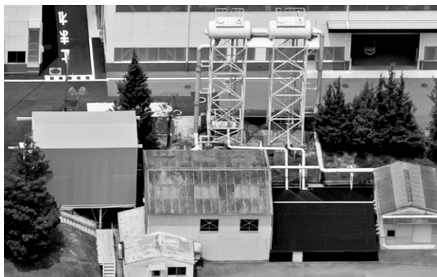
Fig. 3 Panoramic View of Model-Based Test Facility
