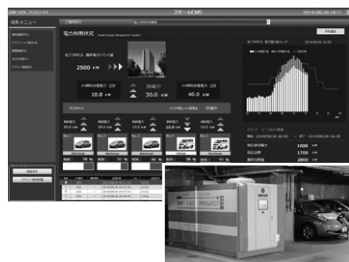
Situation of Power Utilization and Charge/Discharge PCS
